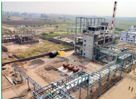
Utility, Common Tank Farm & IB Yard
